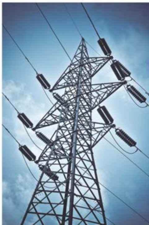
There are 14 concessionaires of electricity operating in São Paulo.
